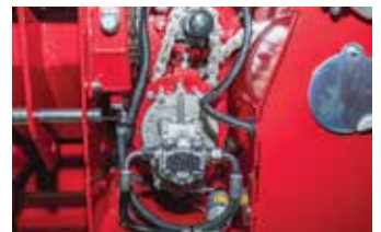
The pump is driven by a cogwheel multiplicator. A pressure filter is installed behind the pump that additionally makes sure that the oil in the system is clean.
